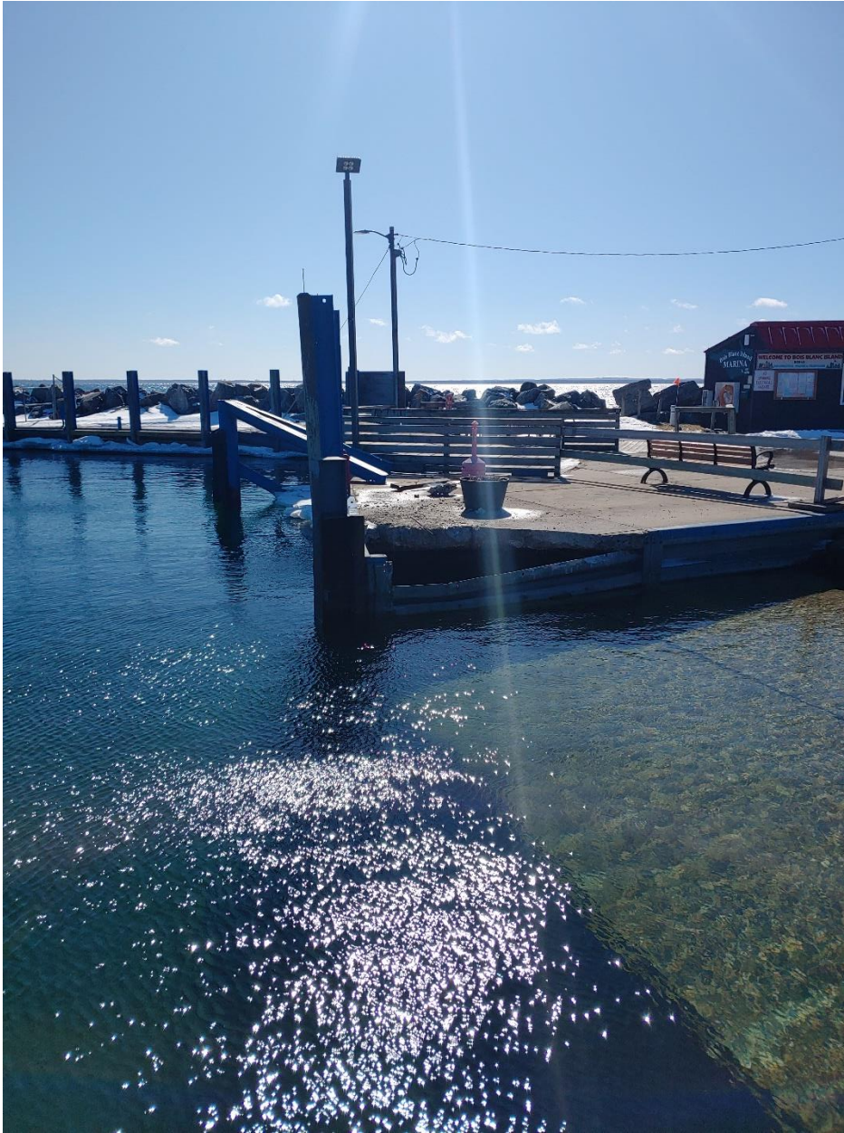
3/10/2020 Damaged structures removed in preparation for the next step of ramp repair.
